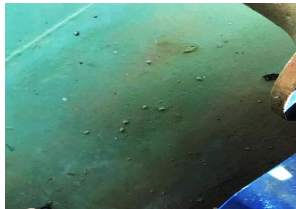
Figure 5: Blister rash on coating of RV-Discovery.
